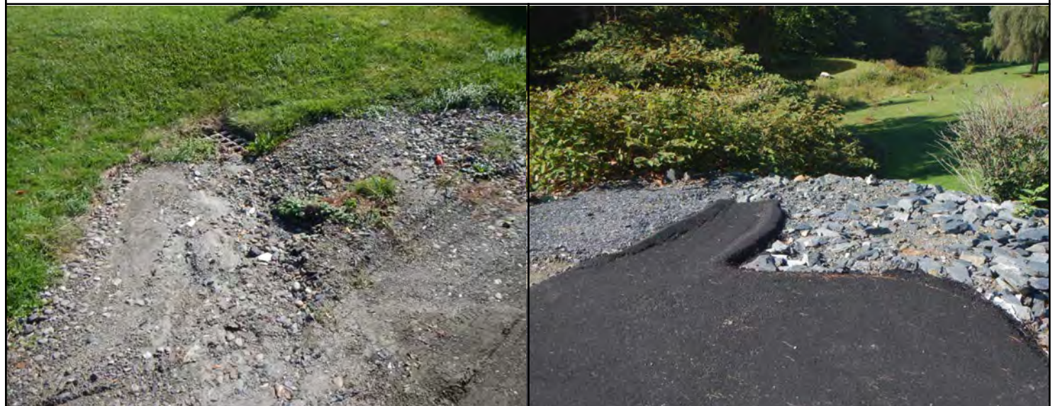
Photo 1. Erosion at catch basin Photo 2. Ineffective turnout structure.
