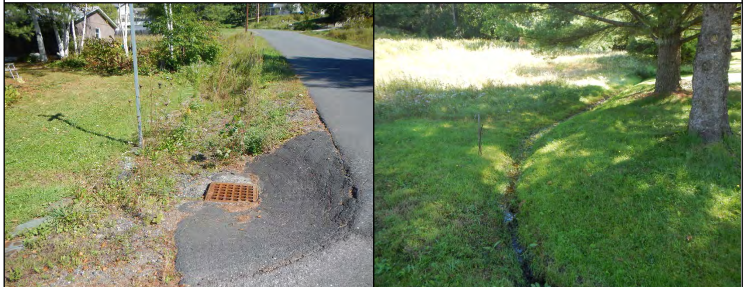
Photo 1. Catch basin and potential treatment area. Photo 2. Narrow ditch that could be reshaped.
