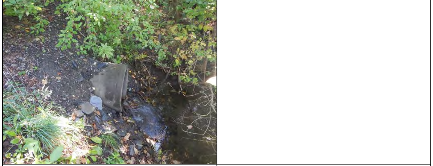
Photo 1. A splash pad at the outfall could reduce localized erosion.
